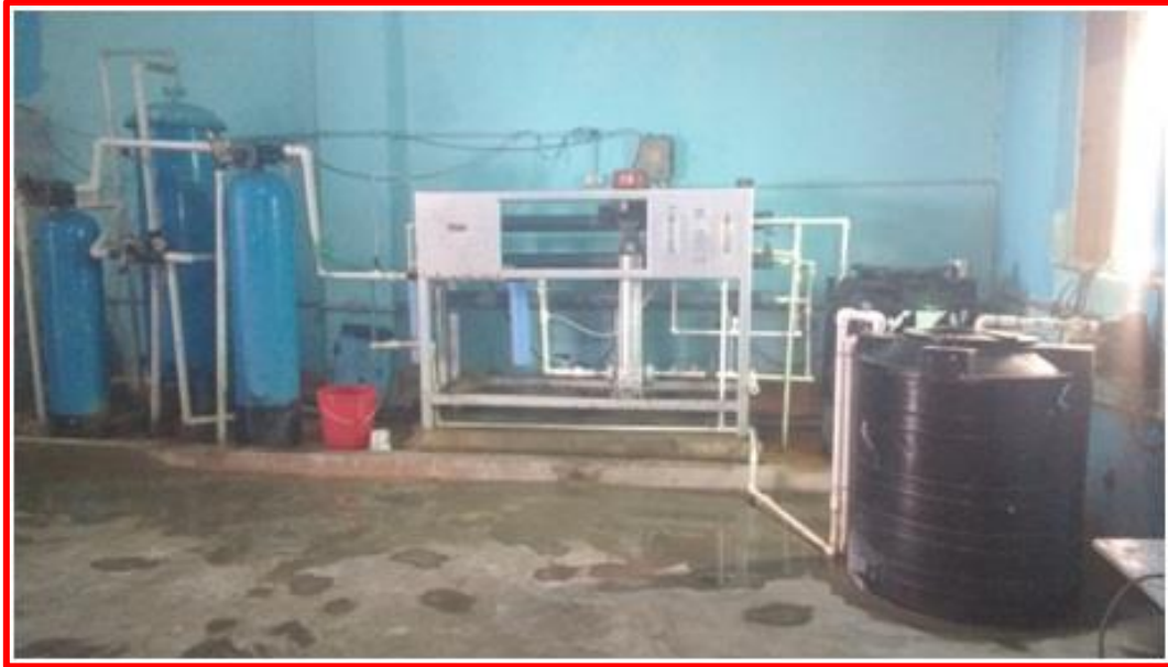
REVERSE OSMOSIS WATER TREATMENT PLANT
